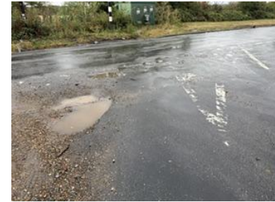
Close up of poor markings, 29 Aug 2026
