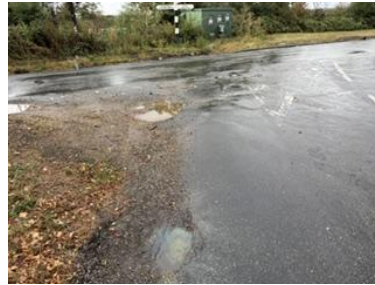
Poor markings, 29 Aug 2026
