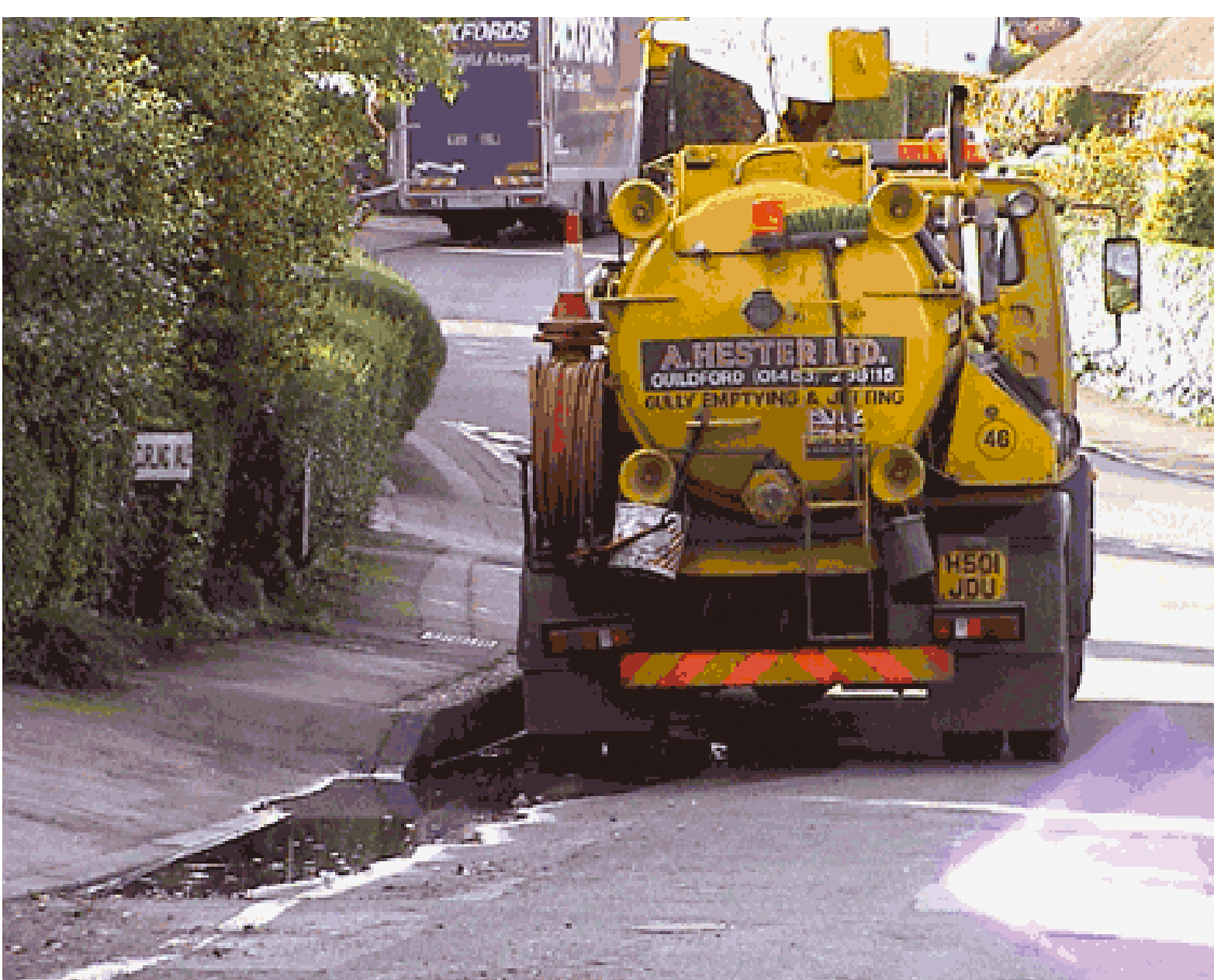
The state of drains
