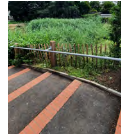
The original surface has been repaired with tarmac, which provides good colour difference between the brick edges, but is not visually pleasing
