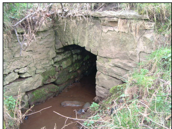
Plate 4. Entrance to a stone culvert at the southwest corner of the field, looking southwest
