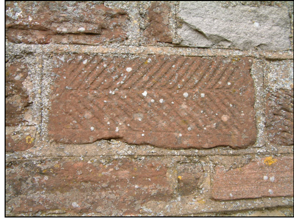
Plate 10. Reused decorated sandstone in the south wall of the modern stable building
