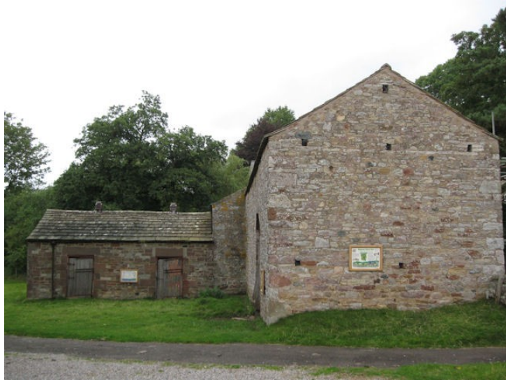
South-facing gable of the Musgrave Church Field Barn – showing the proximity of some of the mature trees around the barn site.
