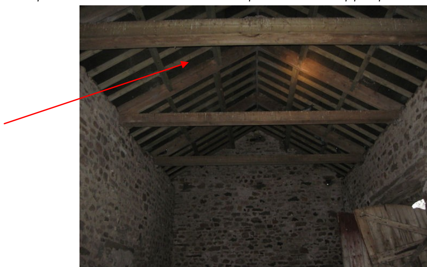
Interior of church barn showing underside of roof, which includes bitumen felt below the traditional stone flagged roof covering.
