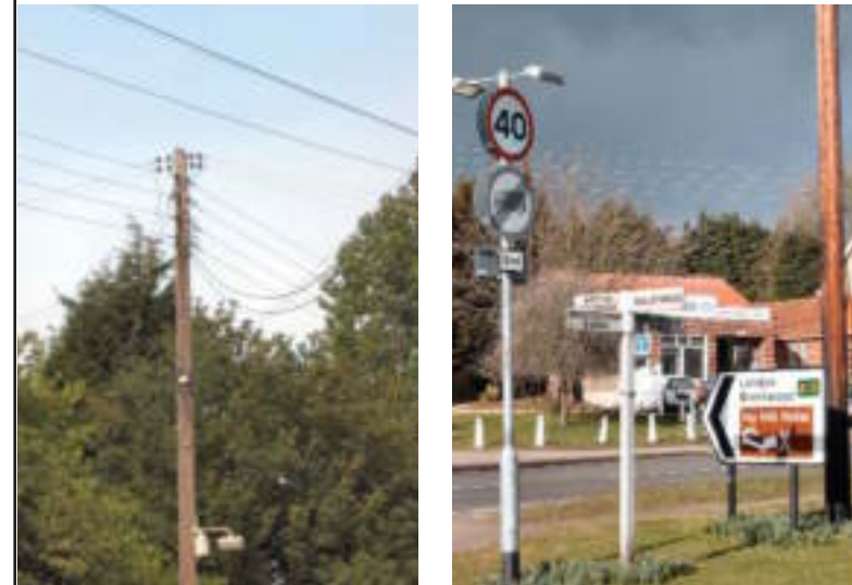
pictured above left: The clutter of overhead cables
