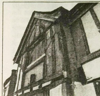
The original jettied front of the Tudor cross wing of 144 Maldon High Street now being exposed
