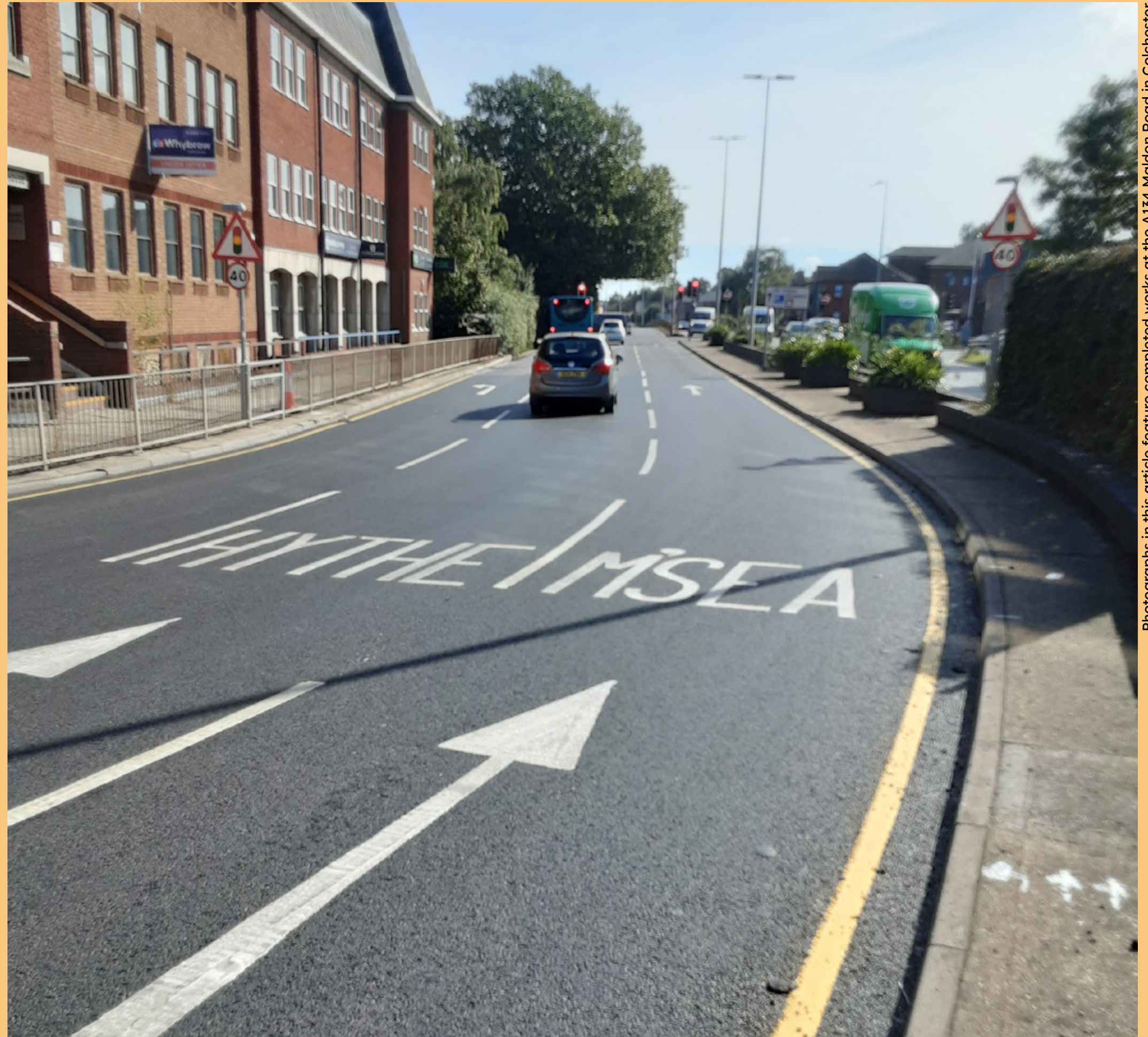
Photographs in this article feature completed works at the A134 Maldon Road in Colchester
