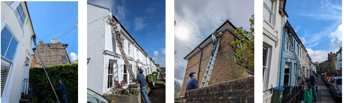
Installing Swift boxes in Abinger Place, Talbot Terrace, and North Way, and an artificial House Martin cup in St. John's Terrace
