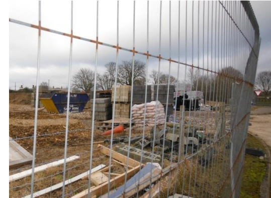
Work has started on eleven new houses on land adjacent to the Museum of Power
