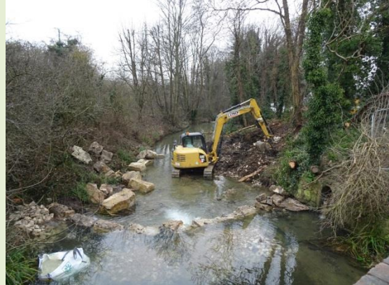
Photograph 2. River restoration: knocking out weirs, the Hogsmill River at bridge along the Tolworth bypass A240, 2015
