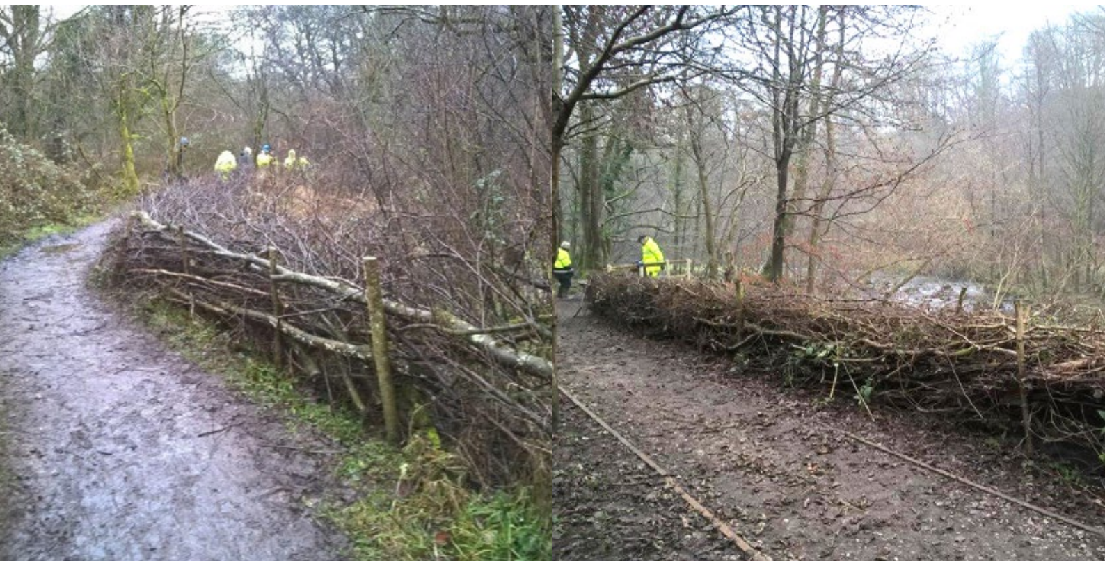
Dead hedging following flood damage in the Brock valley © Wyre Council
