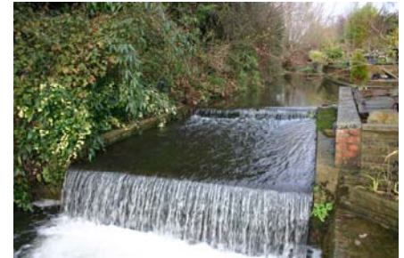
Control Structure on Ems (Wren Centre) d/s Lumley Leat – limits sea trout migration
