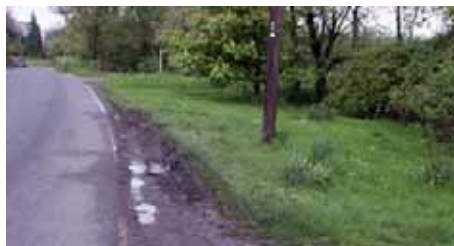
Verge damage in Mill Road
