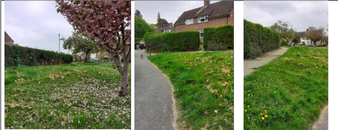
Fig. 1.5.1 Looking south of Footway n.1 showing the poor condition of the concrete slabs and of the existing pedestrian guardrail, also the profile pictures showing the variable slope along it.
