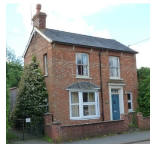
uPVC windows (ground floor) almost never adequately reflect the fine detailing of the glazing bars and sashes of the originals (first floor)
