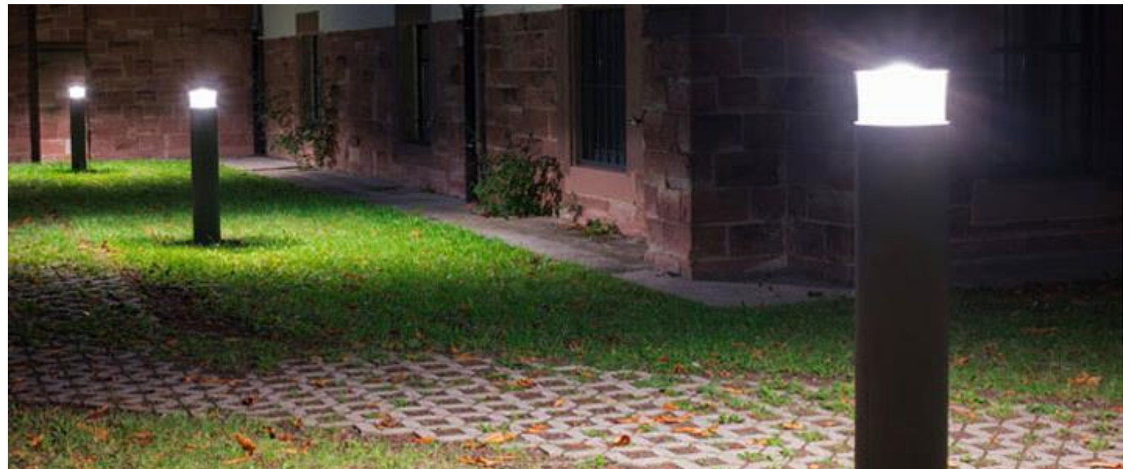
Low level external lighting integrated into the landscape
