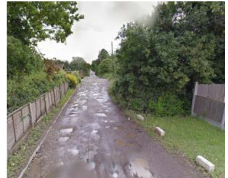
Poor surface water drainage
