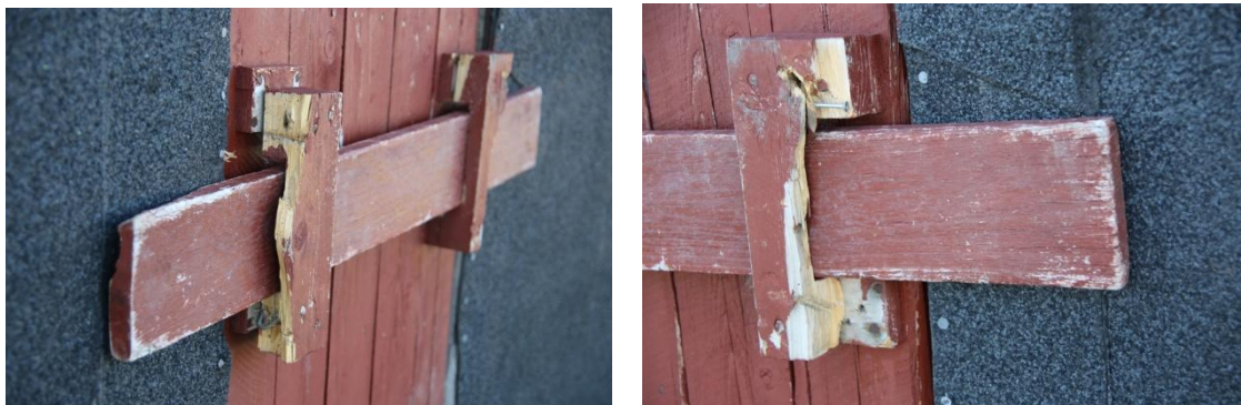
Figure 17: Damage to Kap Pedersens Hut Door
